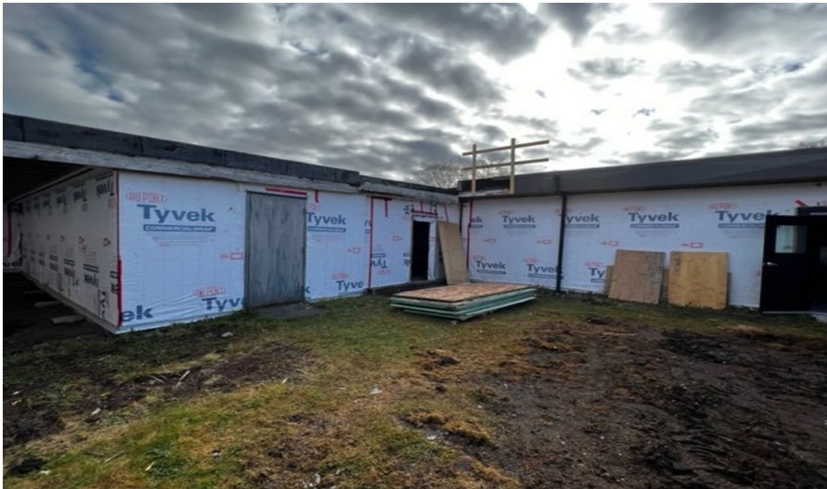
Figure 2 Siding off storage area and ready for demolition, to be replaced with two classrooms
