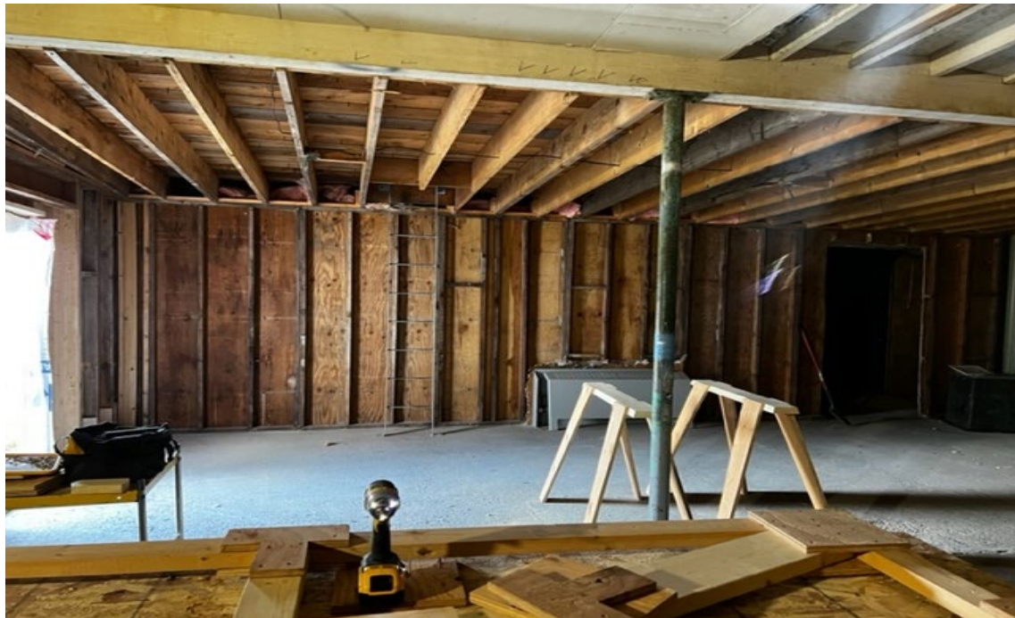
Figure 4 Storage room ready to be demolished to make space for two classrooms
